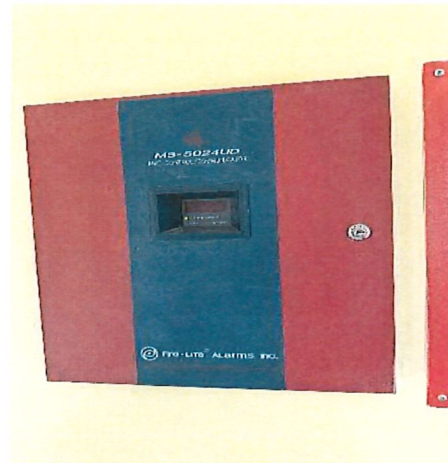
Main Fire Alarm Control Panel
