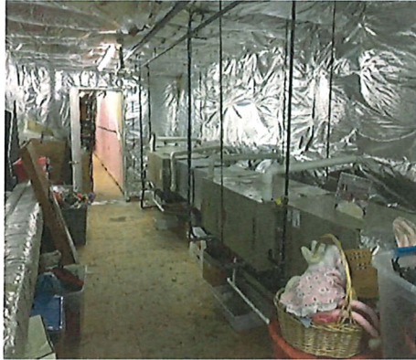
Existing Gas fired Furnaces
