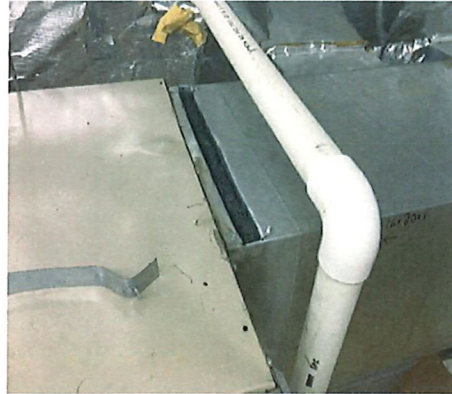
Filter Rack on Existing Furnace
