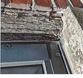
Deteriorated Exterior Wood Trim and Sealant
