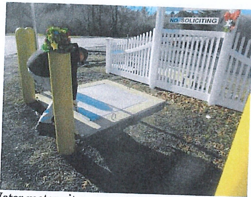
Water meter pit
