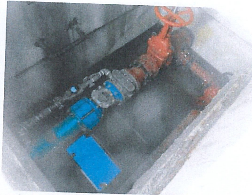
water meter pit and meter, shut off
