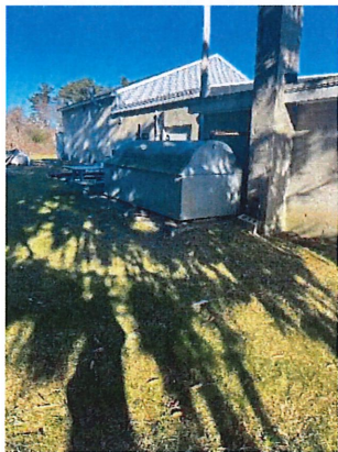
Fuel Oil Tank
