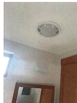
Bathroom Ceiling Fan
