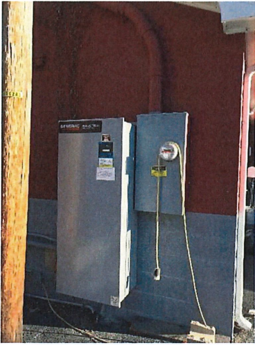
Automatic Transfer Switch
