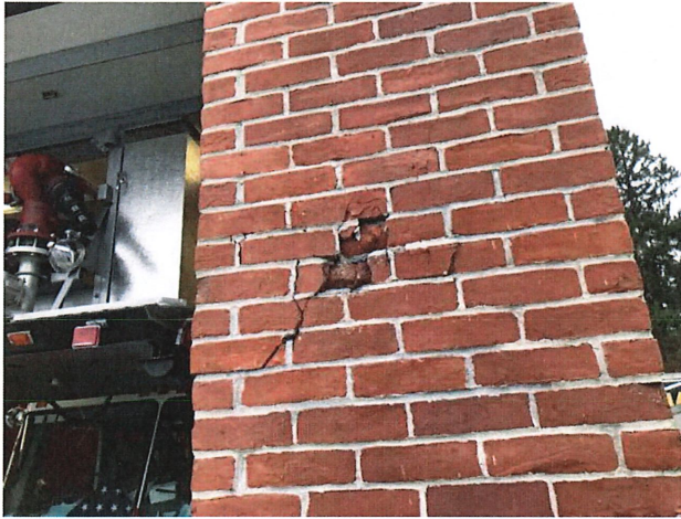
Damage at the front of the bays caused by impacts.
