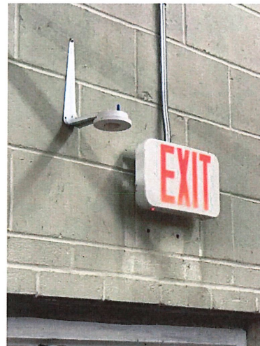
Illuminated Exit Sign
