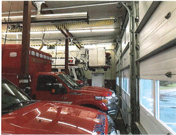
Limited clearance between vehicles and the top/sides of the bay openings.
