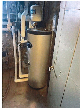
Indirect Hot Water Heater
