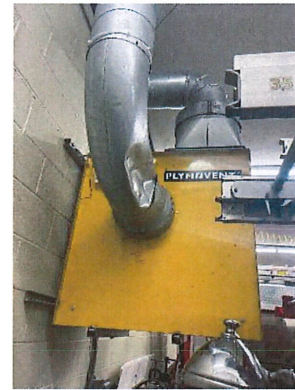
Plymovent – Vehicle Exhaust System
