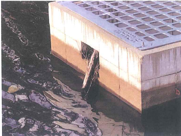
Debris in outlet control structure
