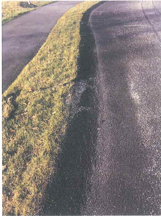
Scarring of bituminous berm
