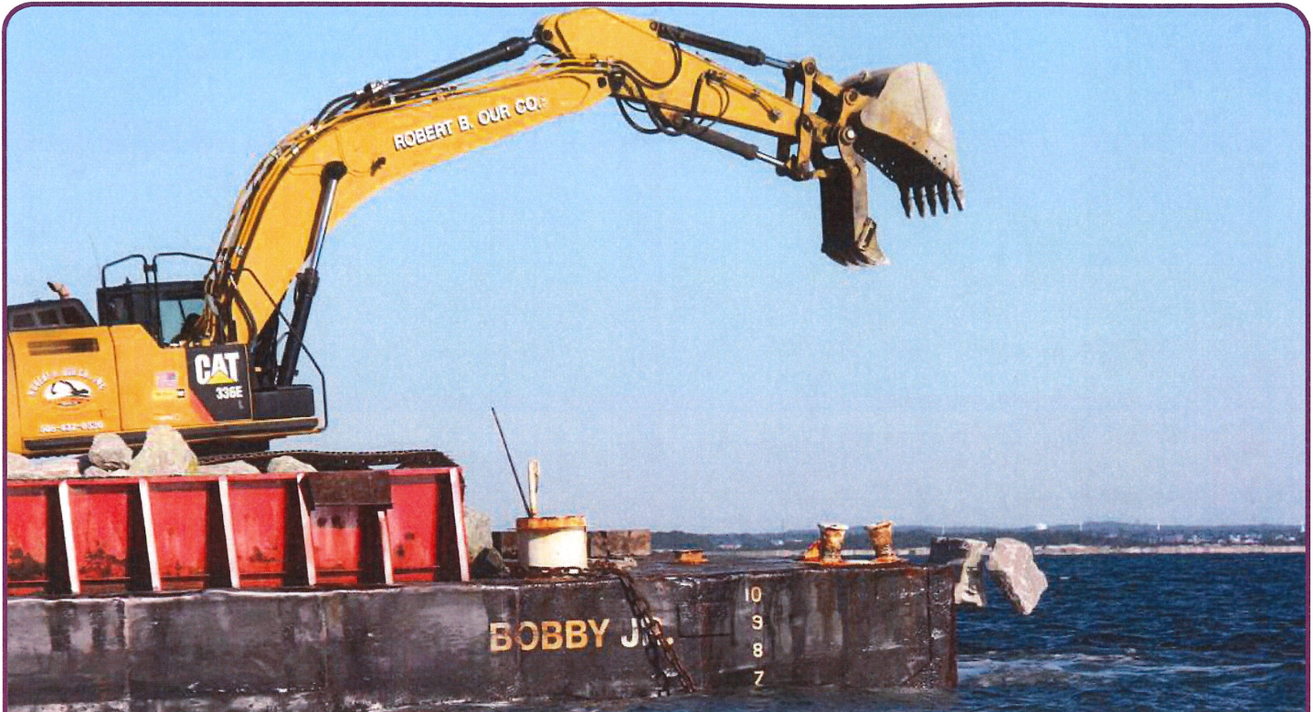
Claw dropping some SCR granite pieces into local waters to build up the reef
