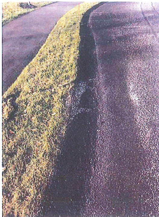
Scarring of bituminous berm
