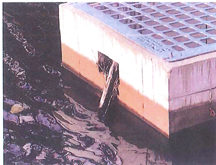
Debris in outlet control structure
